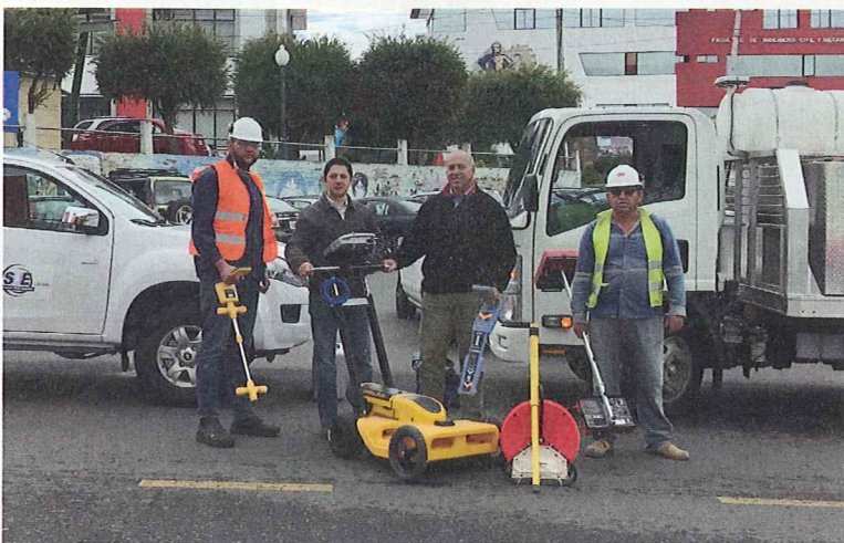
SUE LATAM performs SUE for all of the underground utilities at the Huachi campus of the Technical University of Ambato. Alejandro Rodas, project engineer and General Manager, center left; Nick Zembillas, CEO and recognized international technical expert in SUE, center right.
